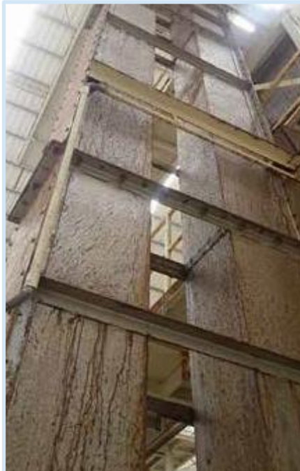
Closed system - cannot be cleaned
