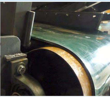
Metal parts conveying
