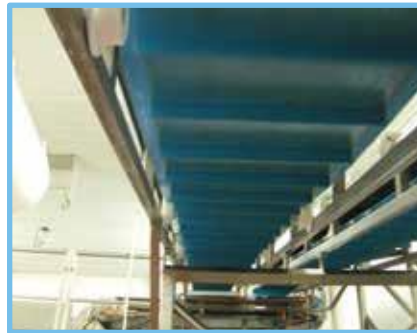
UHMW support on return
