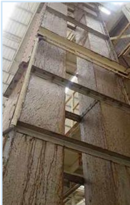
Closed system - cannot be cleaned
