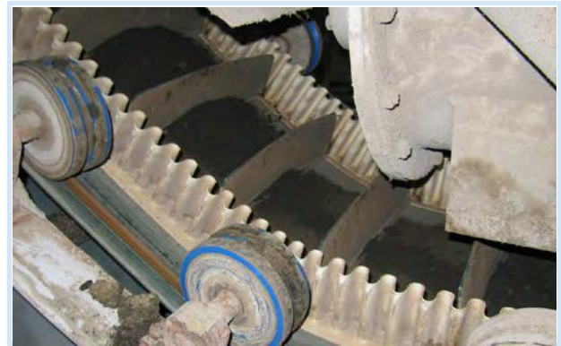
FRG-3 with thermo welded sidewalls and flights: CHEMICAL POWDER (RECYCLED SEWAGE)
